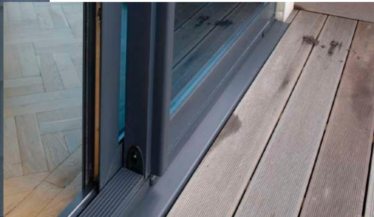
Twin Track Sliding Doors
